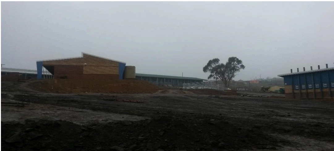
Smuts Ndamase: Construction of new Senior Secondary School – Eastern Cape Value: R59 852 685.00
